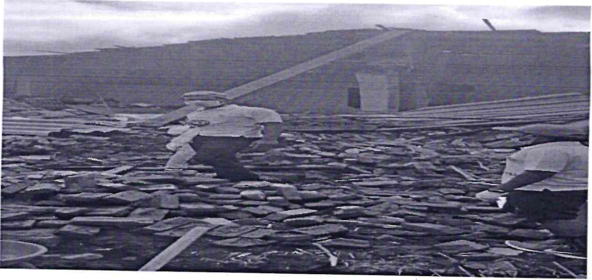
Field work at the flood affected place.
